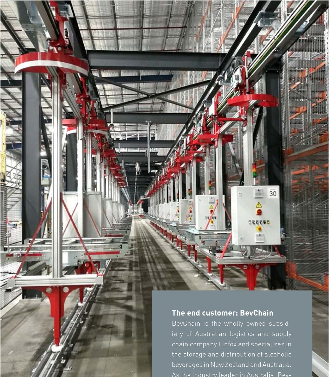
These 37 intelligent vehicles receive their orders via a static head control. They find their way by scanning barcodes on the system.
